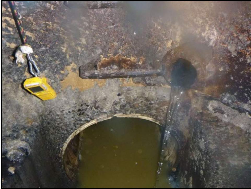
Monitored NW Influent Pipe
