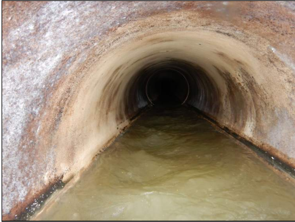
Monitored N Influent Pipe
