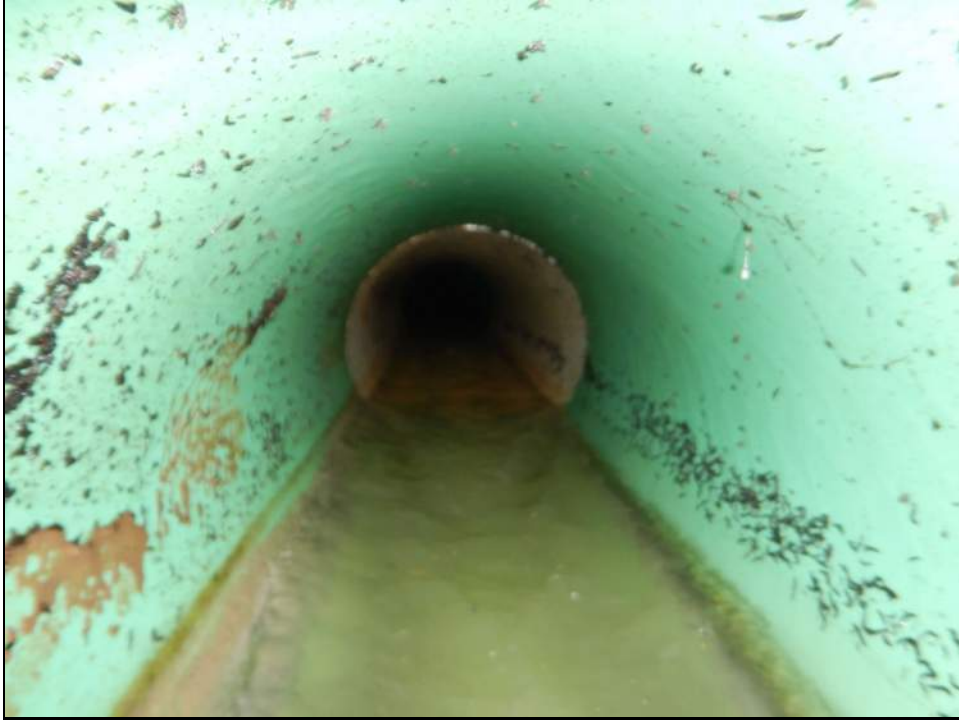
Monitored W Influent Pipe
