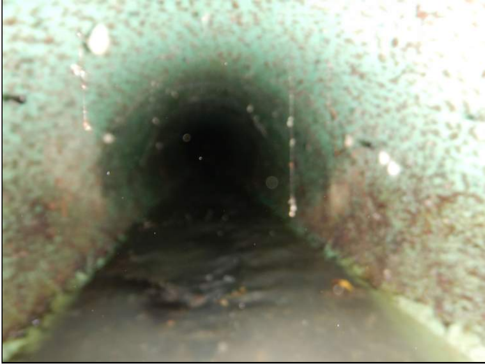
W Influent Pipe
