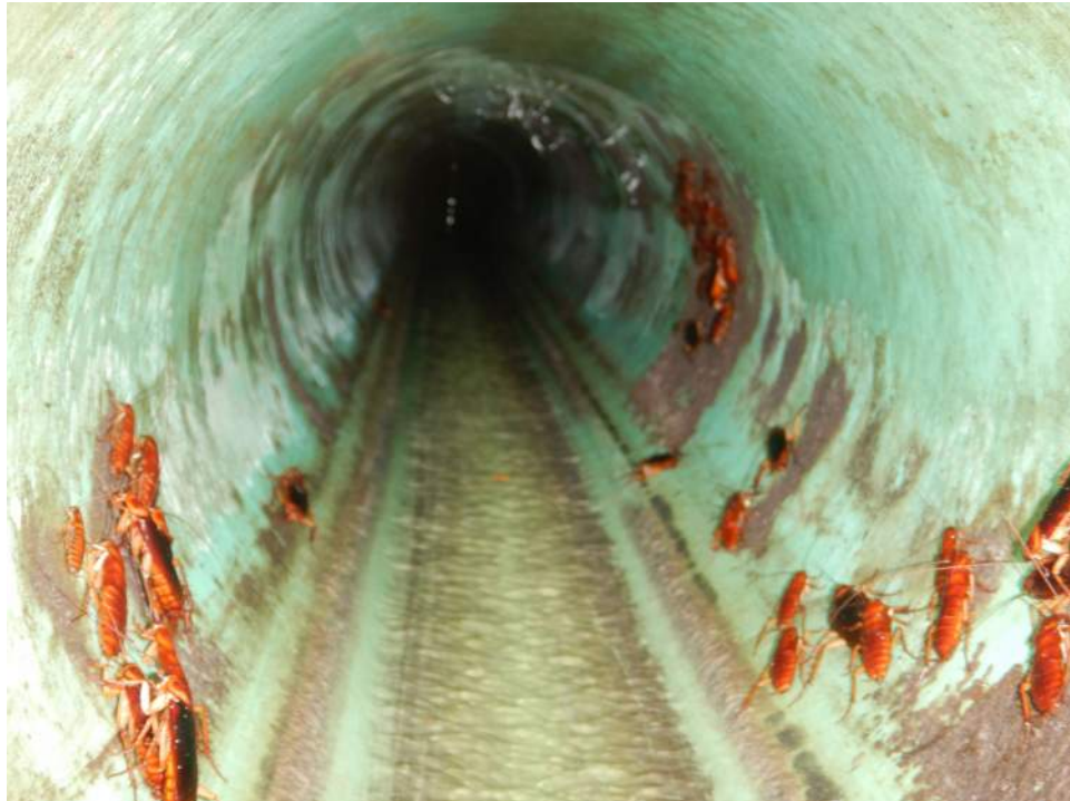
Monitored N Influent Pipe
