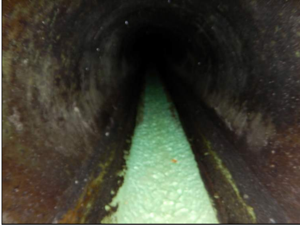
W Influent Pipe
