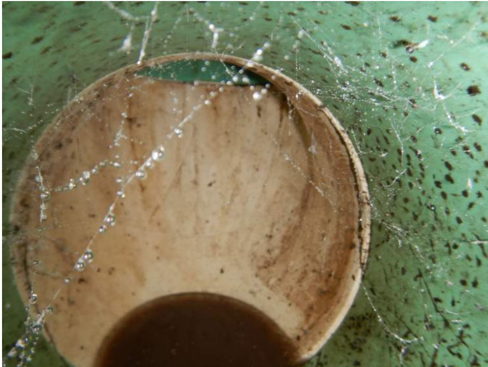
E Low Influent Pipe
