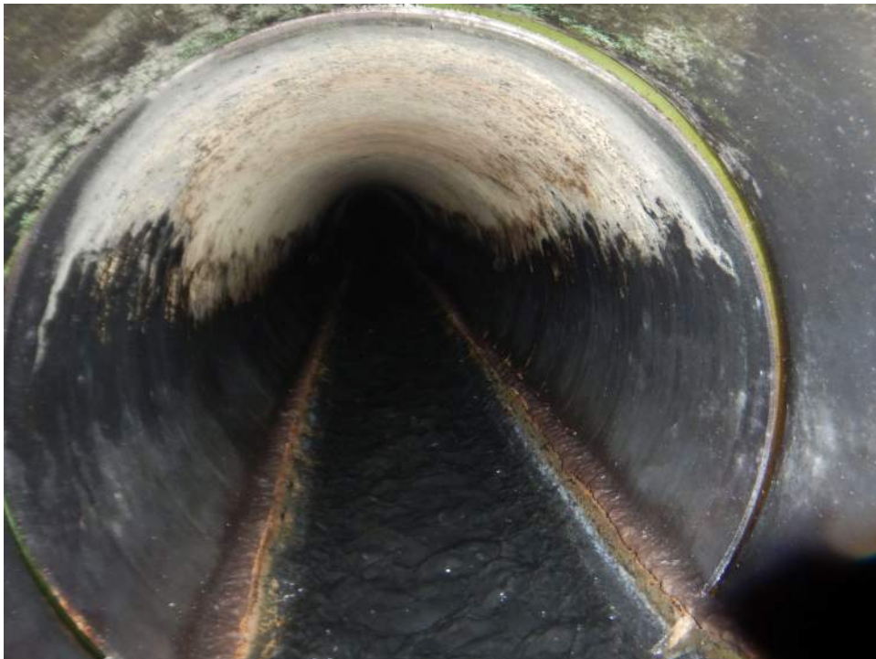
Monitored NE Influent Pipe
