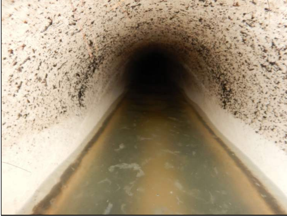
Monitored N Influent Pipe
