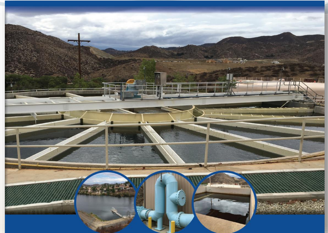
Image of the CLWTP clarifier
