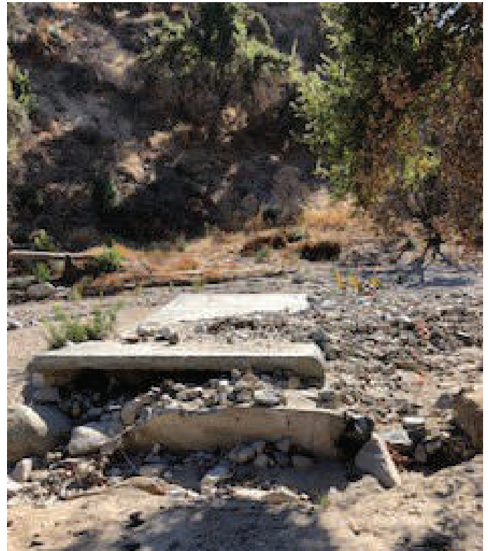
Existing Arizona crossing that is damaged and will be replaced will have streambed impacts that will require mitigation
