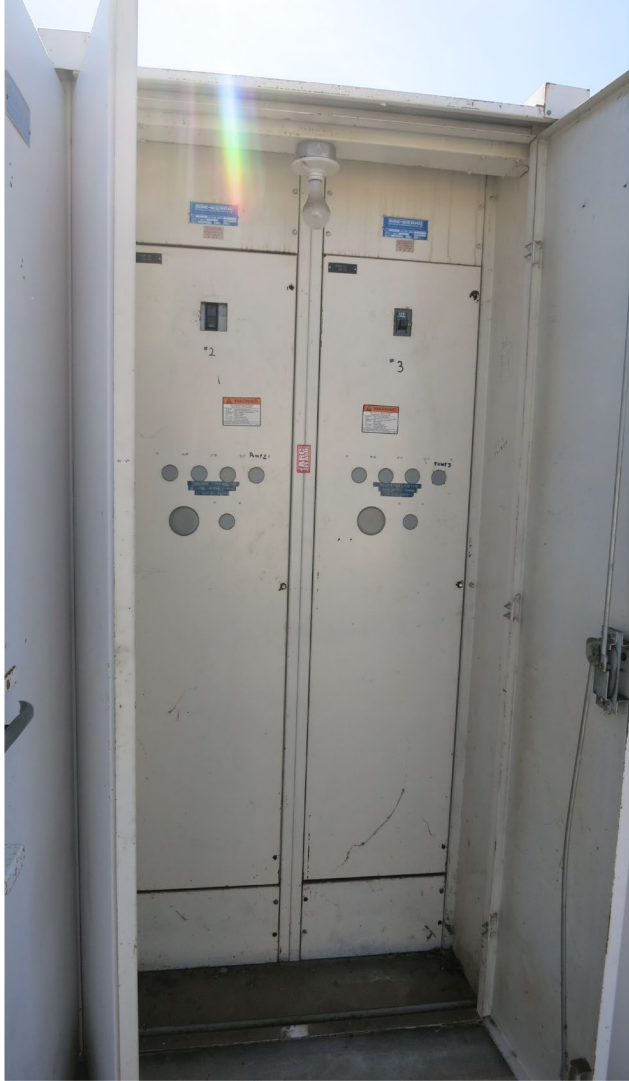
GRAND AVE BOOSTER STATION
