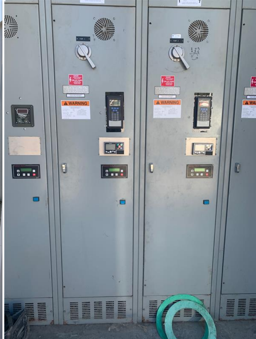
COTTONWOOD BOOSTER STATION
