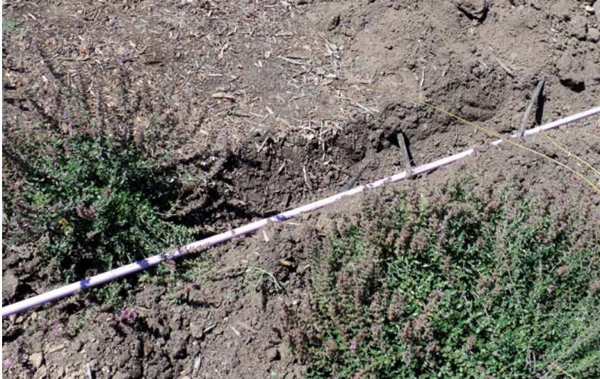
Inline emitter tubing being installed a couple inches below ground. Courtesy of Camrosa Water District.
