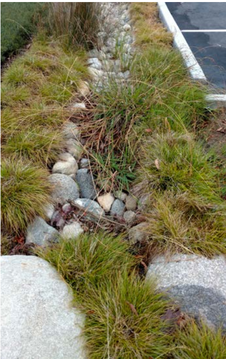
A colony of crabgrass has taken root in this rocky swale. If not removed, the crabgrass might affect the flow of water and cause unwanted pooling elsewhere.
